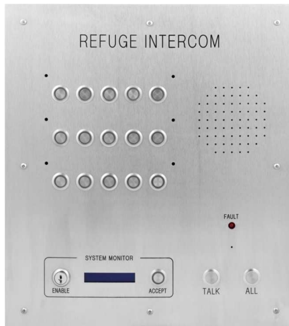
Fig 11:25 Standard System Fifteen Way Master Station
